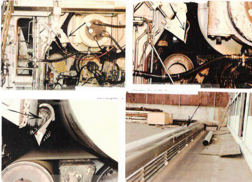
Lazy Steam Injector with retraction mechanism installed on Norpac #1 in 1980
